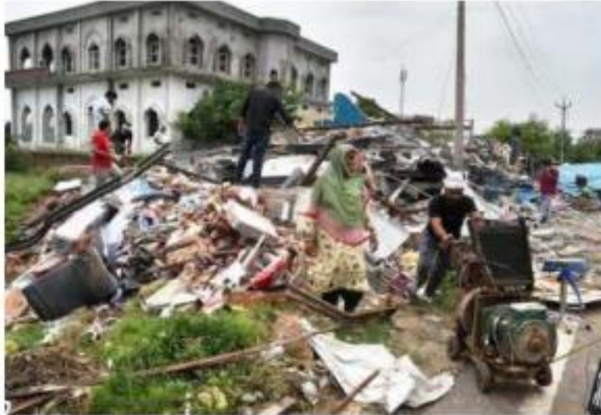
Razed: 'Illegal constructions' being demolished in violence-hit Nuh district on Saturday. SUSHIL KUMAR VERMA
