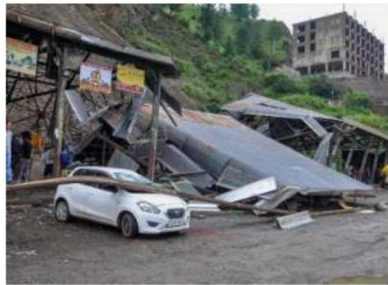
Squashed in rain: Damaged sheds of the Bhattakufer apple market after a landslide due to heavy monsoon rainfall, in Shimla. PTI
